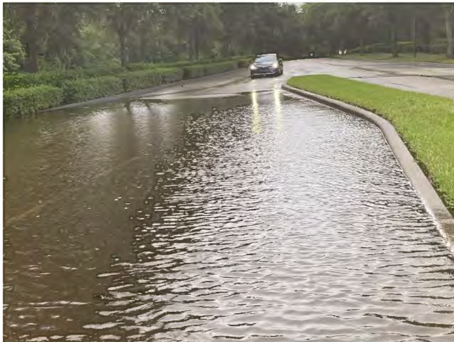
Looking south along Cotillion Blvd exit lane – water flooding street.
